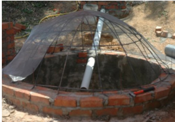
Fig. 15. Mesh network that supports the gas holder of a household unit
