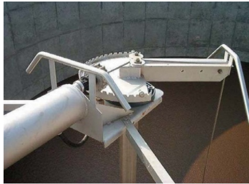
(b) Cable and gear protection system
