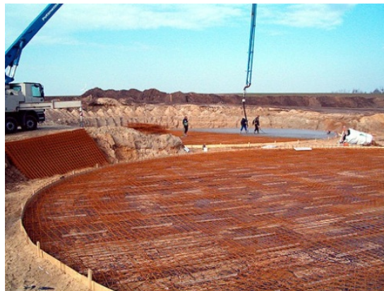
Fig. 8. Structuring the grid irons for a commercial biogas plant (MT-ENERGIE GmbH & Co. KG)
