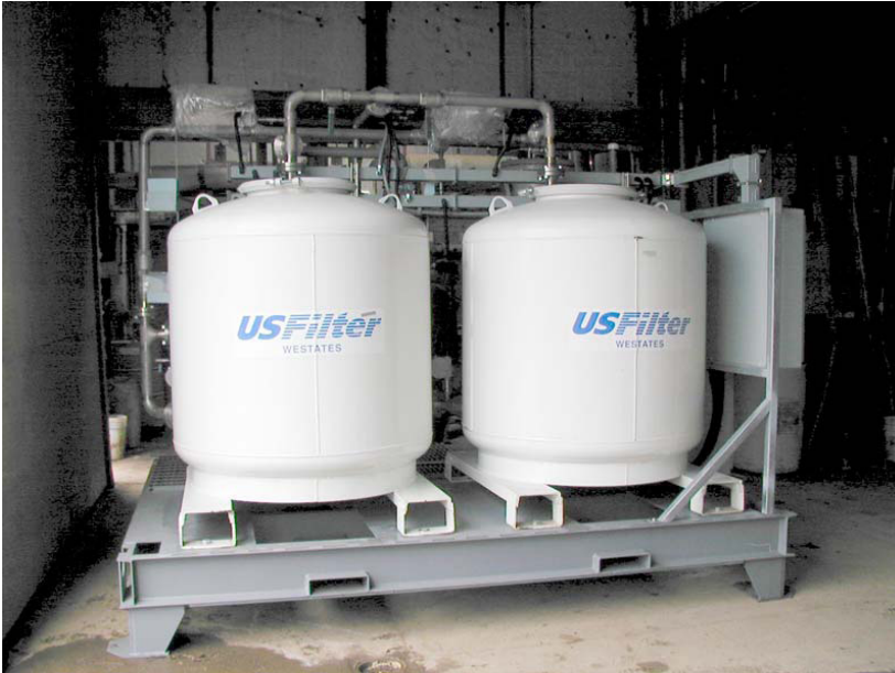
Fig. 19. Activated carbon beds of the GPU (Chandrasekar, 2006)
