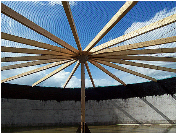
Fig. 14. Wood structure and mesh network that supports the gas holder of digester in a commercial biogas plant (MT-ENERGIE GmbH & Co. KG)
