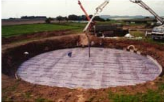
Fig. 9. Pouring the concrete mixture for a commercial biogas plant (BIOGAS NORD GmbH)
